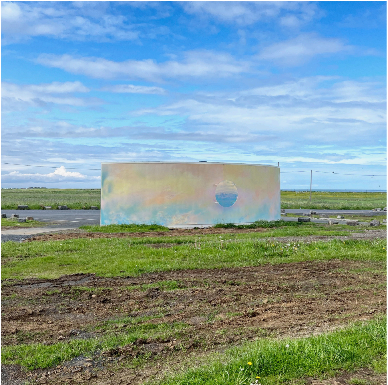
Figure 2. Seltjarnarnes Heating Company - Pumping Station SN-12 . All images by author unless otherwise noted.
